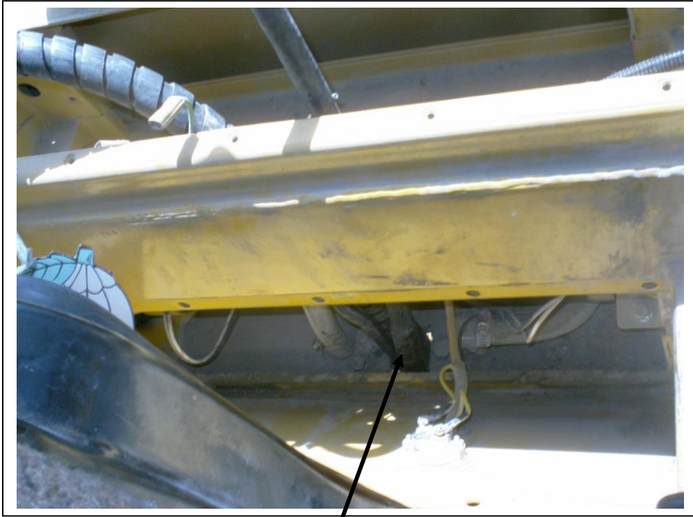
A/C hoses and wiring coming up through the floor of the cab.
